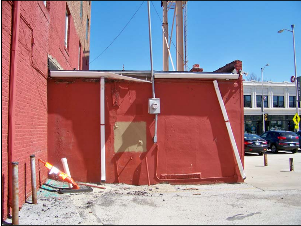
3634 Main St – looking east – deterioration of gutter, downspouts; failure of finishes
