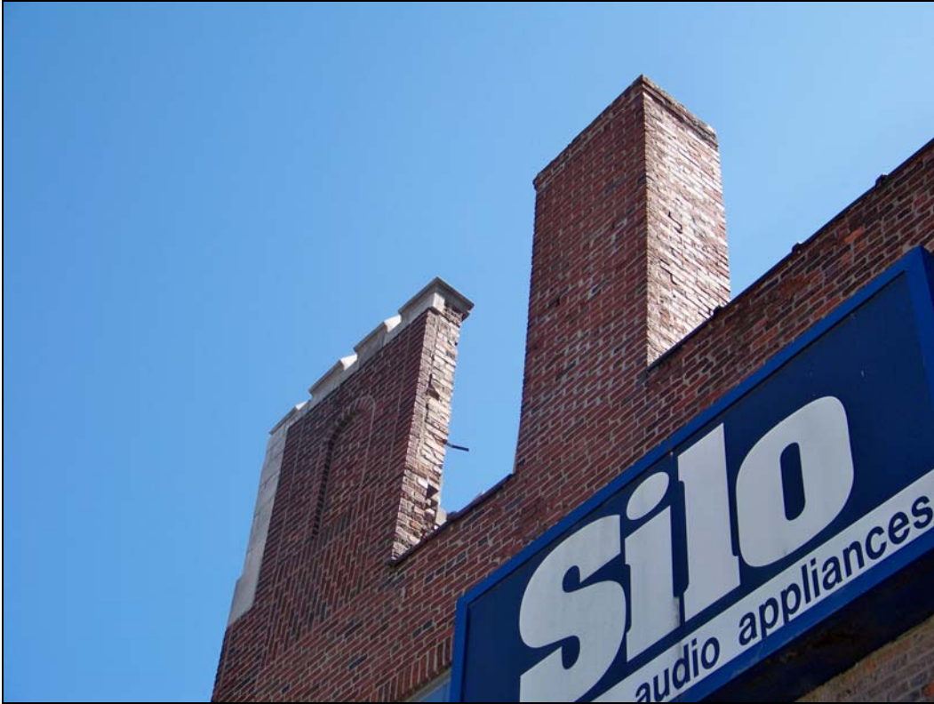
3620 Main St – looking south – deterioration of parapet wall, mortar, masonry
