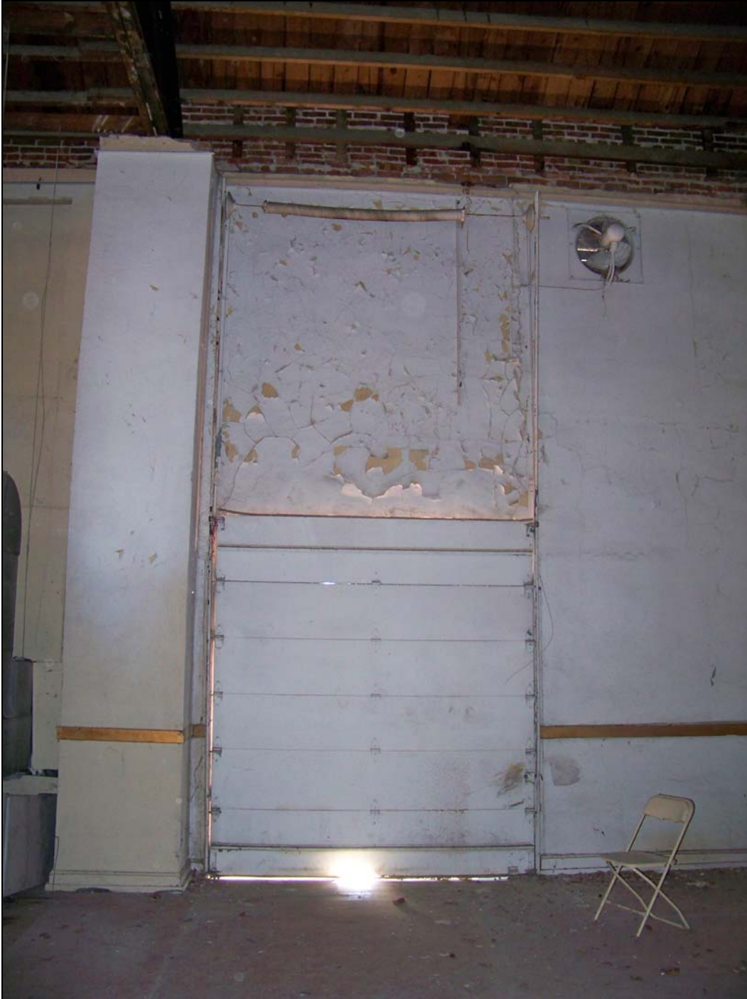
3620 Main St – interior – deterioration of door; failure of finishes
