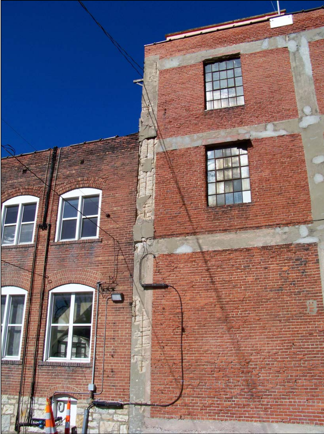
3240 Main St – looking north – deterioration of concrete structure, windows, roof coping
