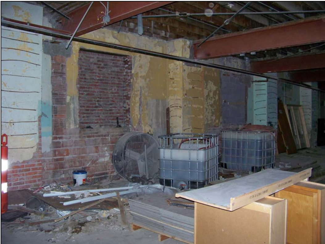
3620 Main St – interior – trash/debris
