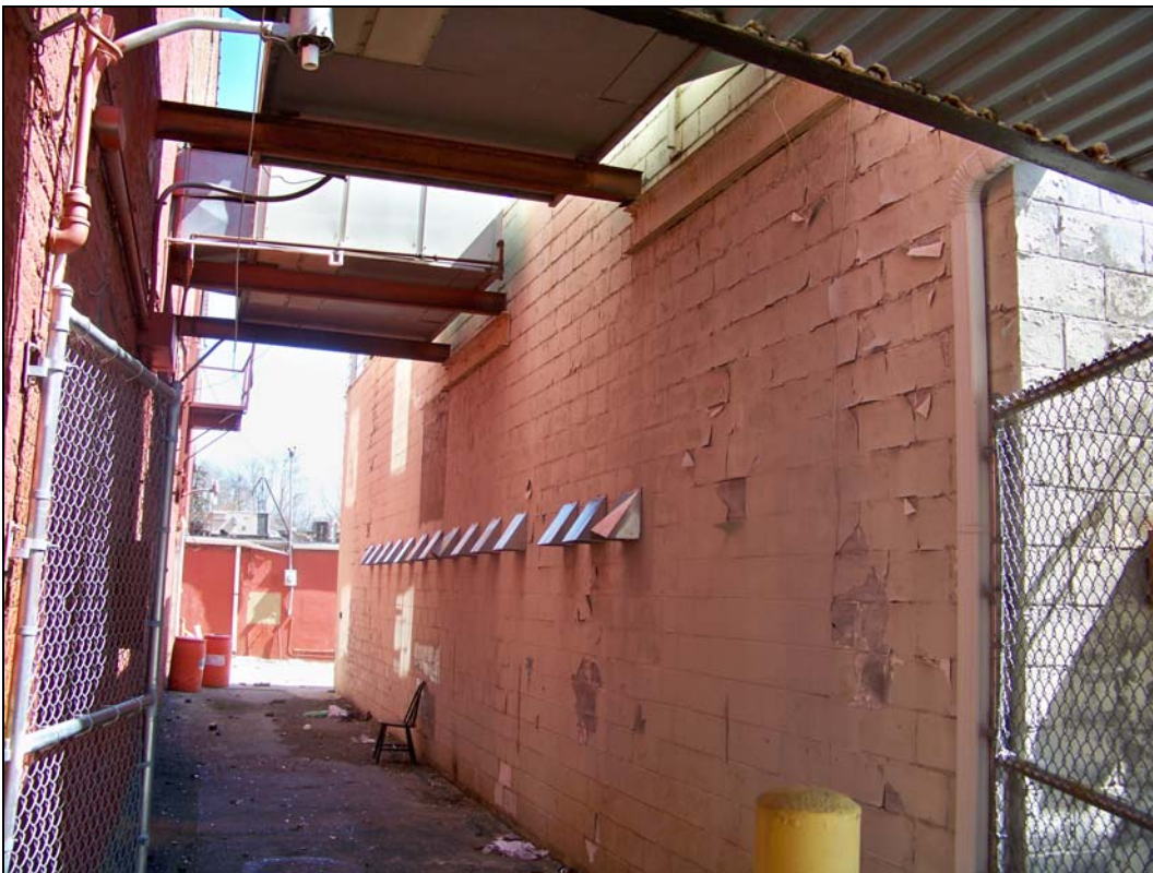
3634 Main St – looking east – failure of finishes
