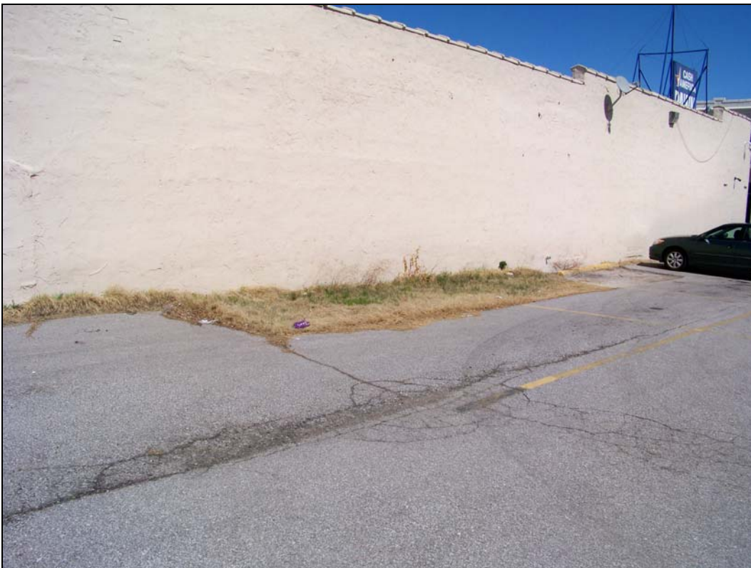
2 W. 37 th St – looking north – deterioration of parking surface
