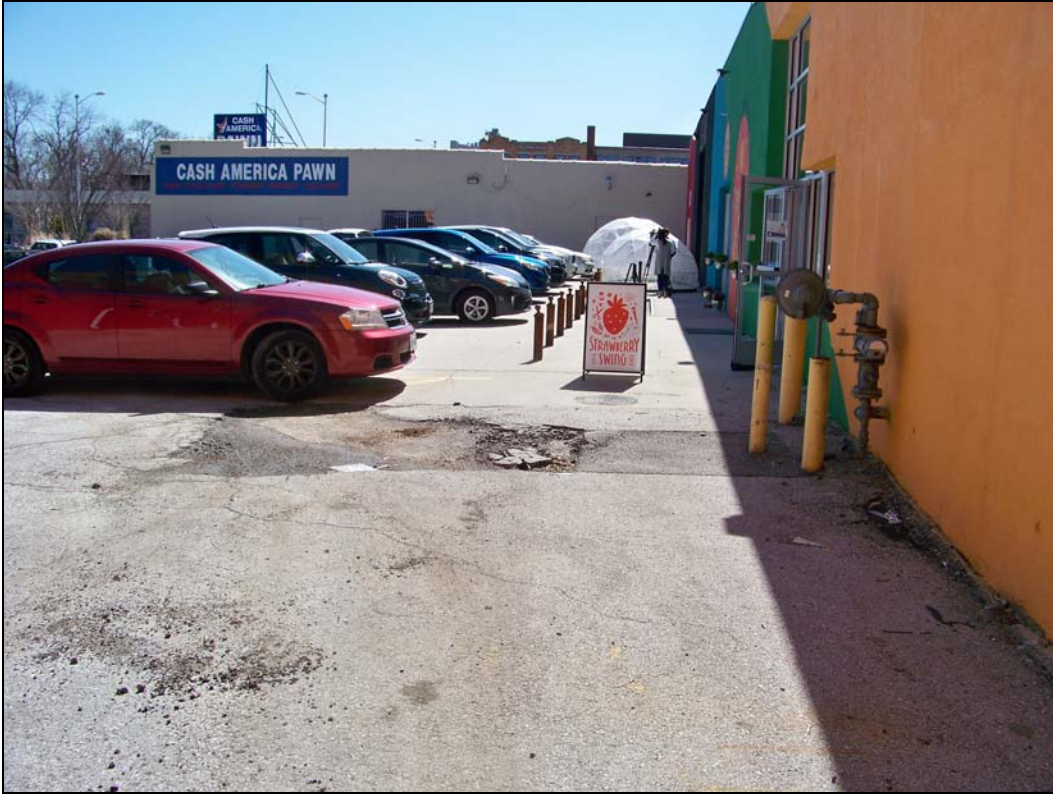
3634 Main St – looking south – deterioration of pavement
