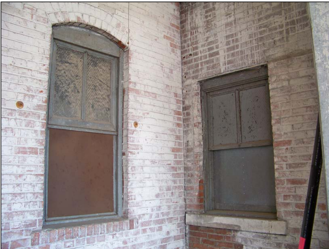
3244 Main St – looking northeast – deterioration of windows; failure of finishes
