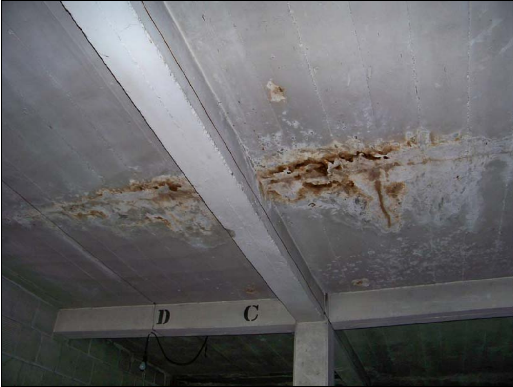
3244 Main St – interior – deterioration of concrete structure; water damage, corroding steel rebar
