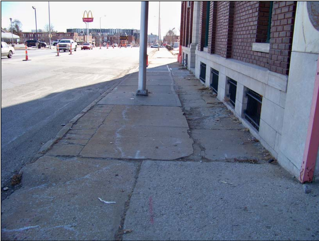
3244 Main St – looking south – deterioration of sidewalk
