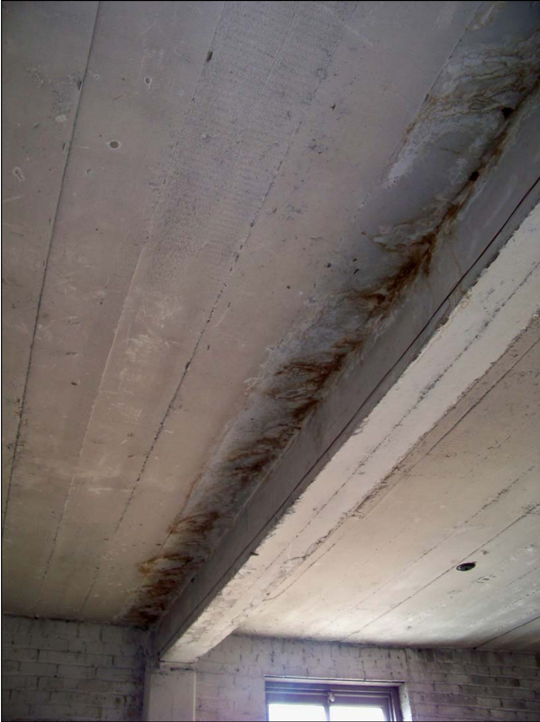
3244 Main St – interior – deterioration of concrete structure; water damage, corroding steel rebar
