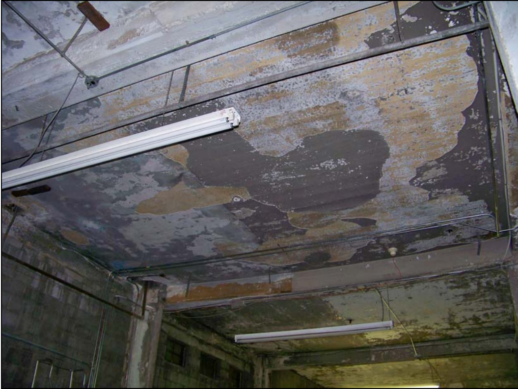
3240 Main St – interior – failure of finishes
