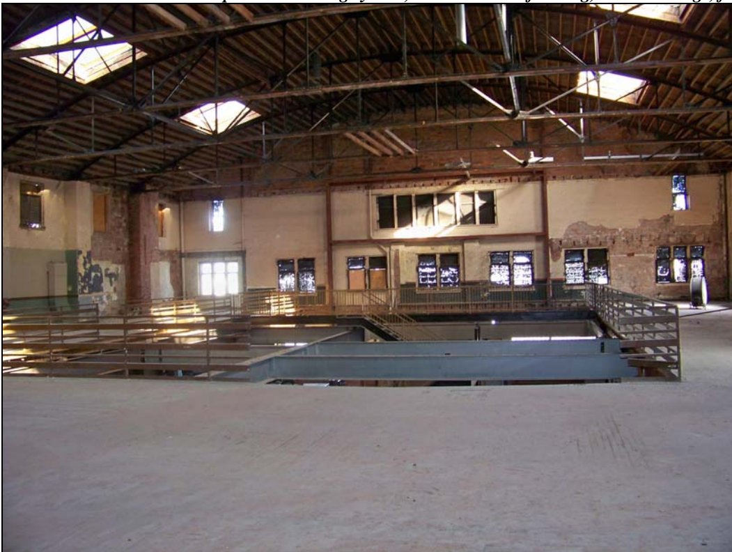
3620 Main St – interior – lack of railing
