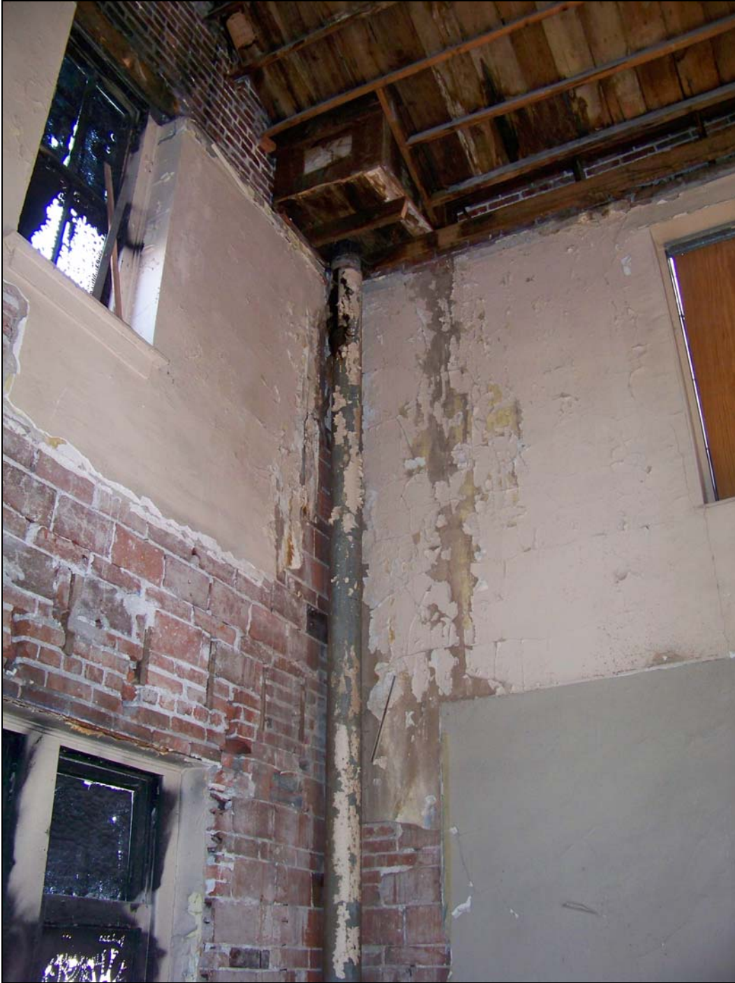
3620 Main St – interior – deterioration of windows; failure of finishes; evidence of water intrusion
