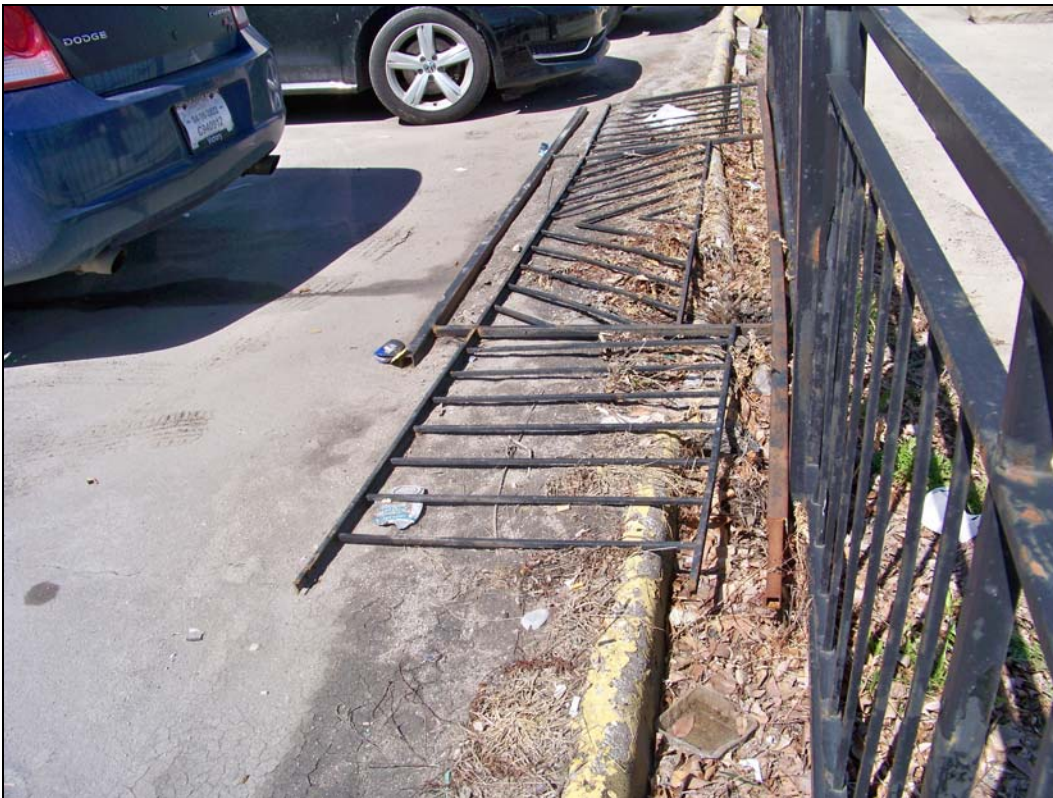
2 W. 37 th St – looking north – deterioration of fence, wheel stops
