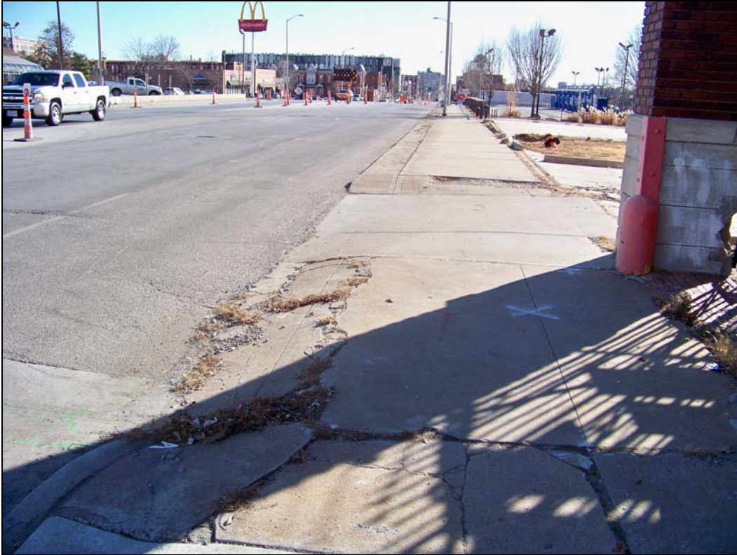
3244 Main St – looking south – deterioration of sidewalk
