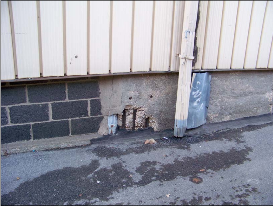
3240 Main St – looking south – deterioration of wall, downspout
