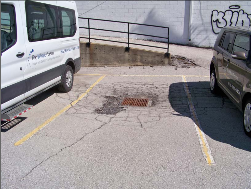
3633 Baltimore Ave – looking east – deterioration of pavement
