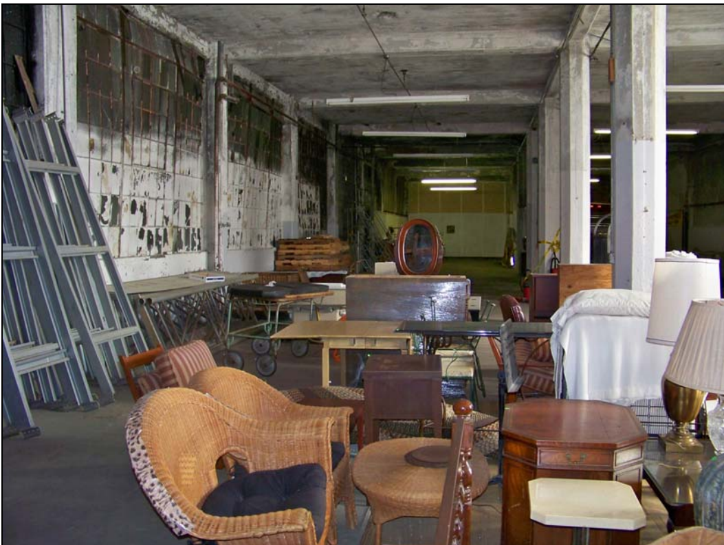
3240 Main St – interior – deterioration of windows; failure of finishes
