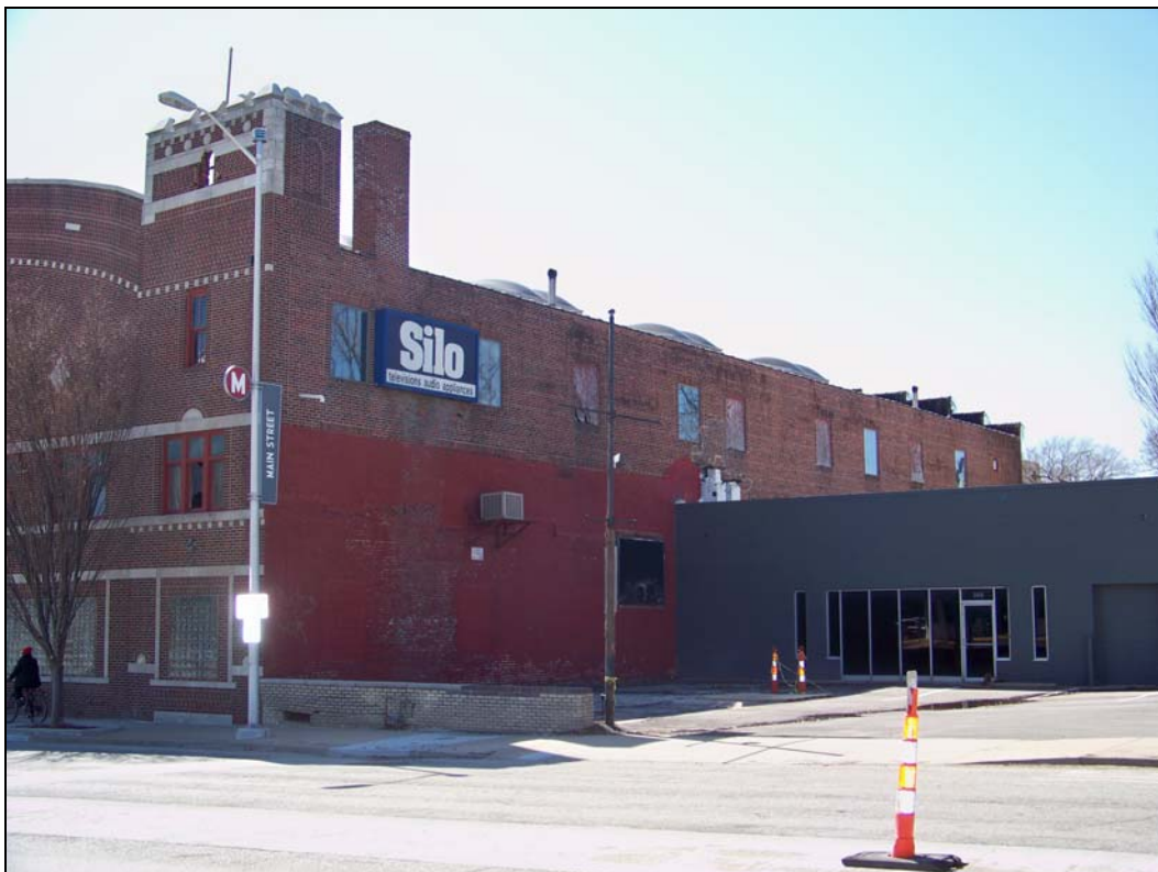
3620 Main St – looking southwest – deterioration of windows; failure of finishes
