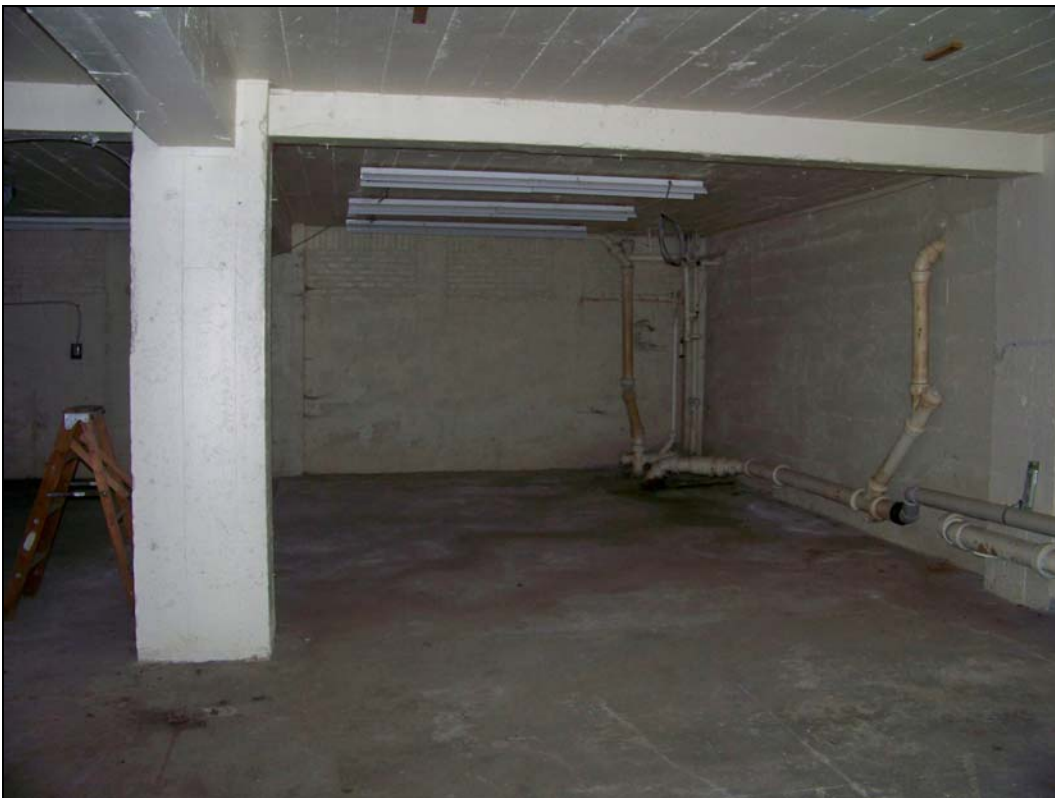
3240 Main St – interior – leaking plumbing and staining of floor
