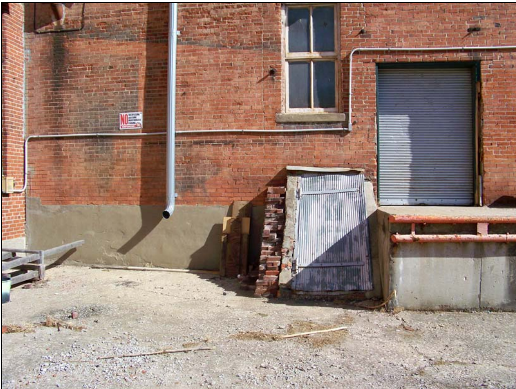
3244 Main St – looking east – deterioration of doors, pavement; failure of finishes
