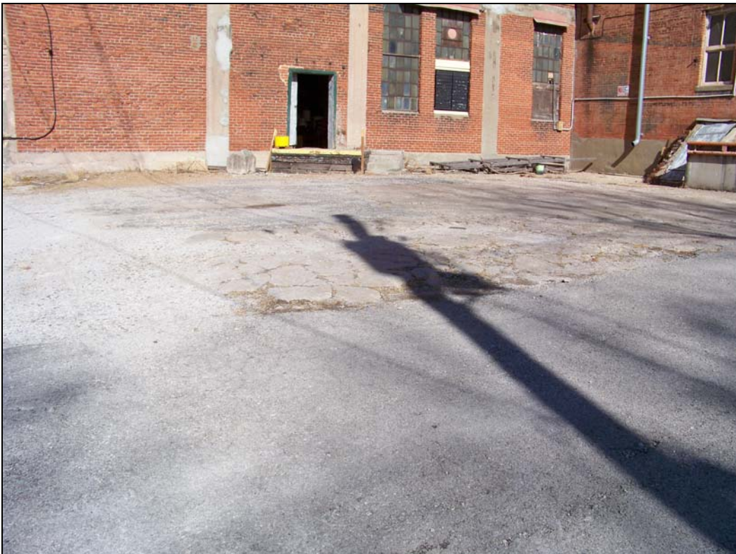
3244 Main St – looking northeast – deterioration of pavement
