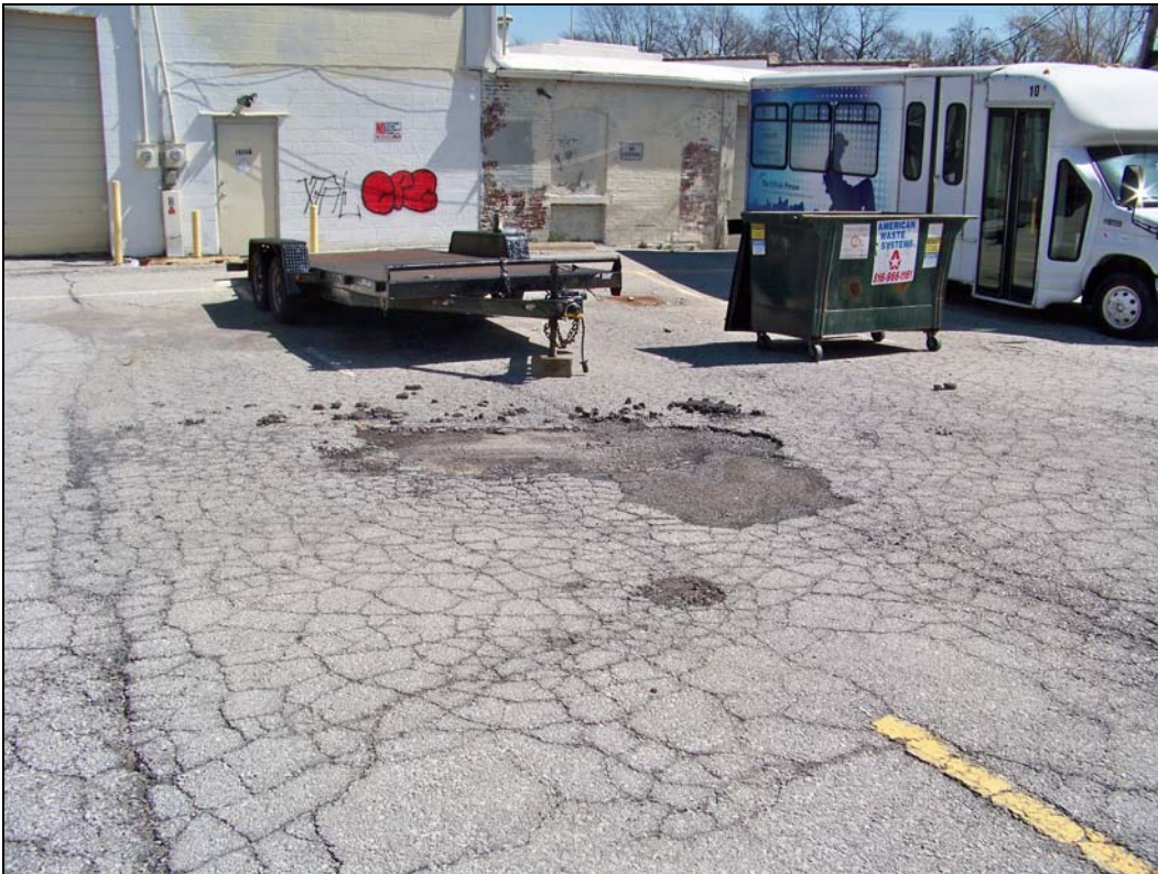
3633 Baltimore Ave – looking east – deterioration of pavement
