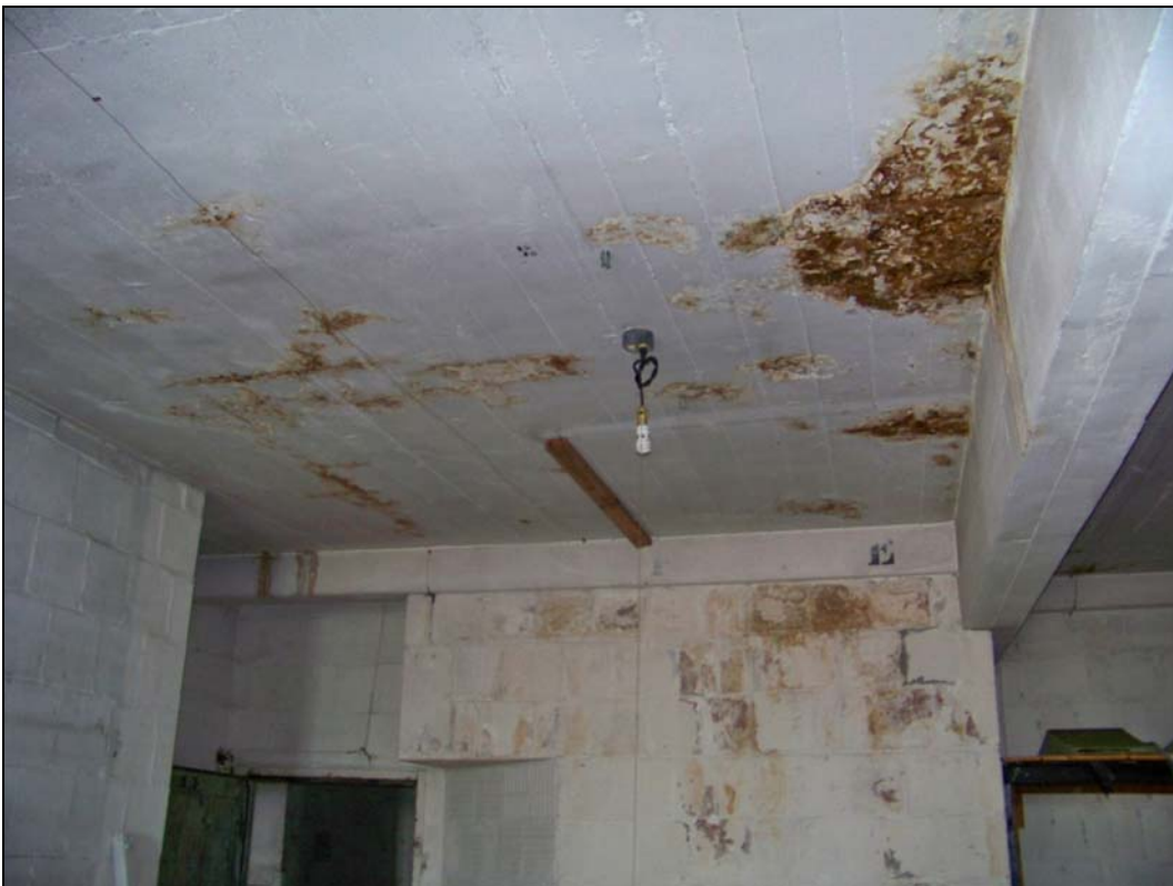
3244 Main St – interior – deterioration of concrete structure; water damage, corroding steel rebar
