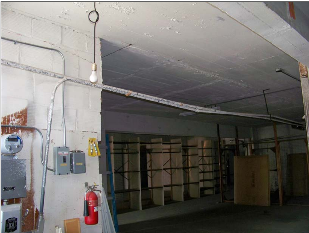
3244 Main St – interior – low-hanging electrical conduit
