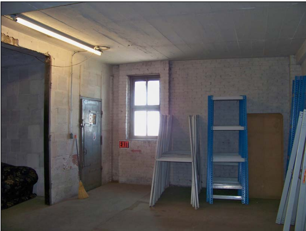
3244 Main St – interior – lack of emergency/life safety lighting
