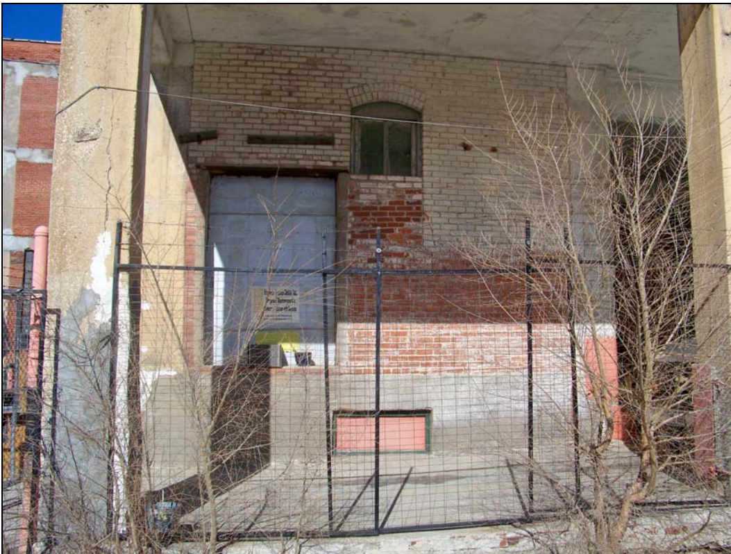
3244 Main St – looking north – failure of finishes; deterioration of door, windows
