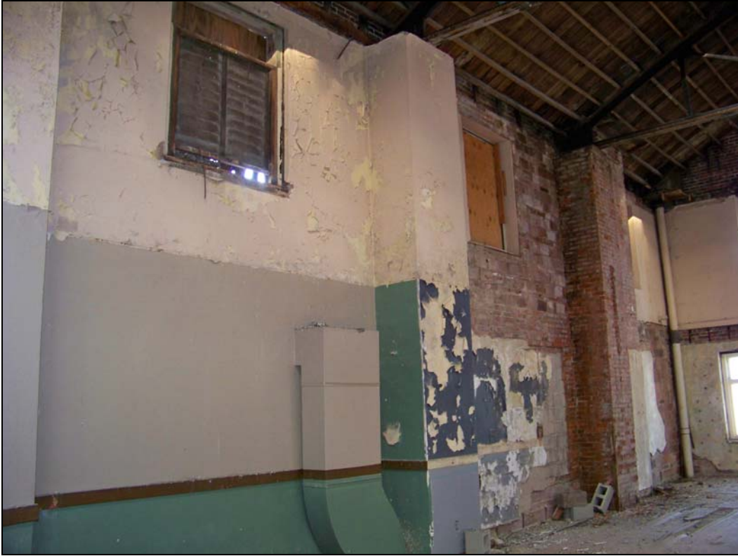
3620 Main St – interior – failure of finishes; deterioration of windows, vents; inoperable HVAC
