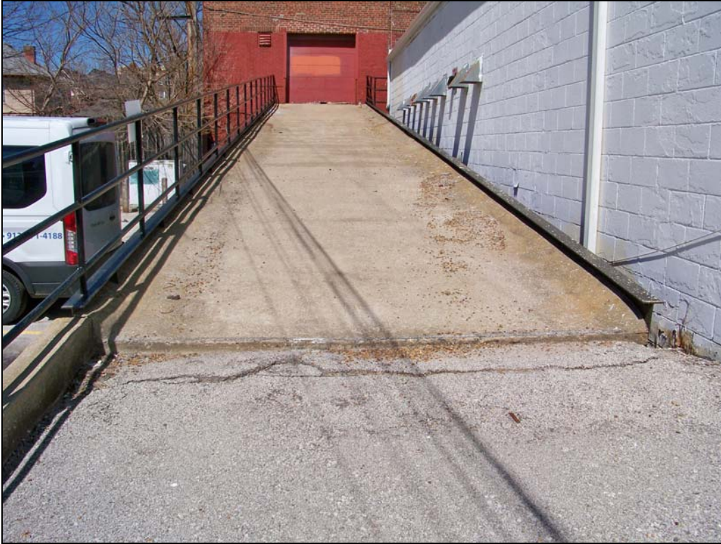
3634 Main St – looking north – deterioration of pavement
