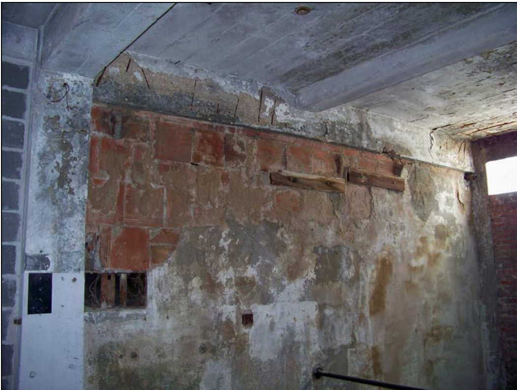
3240 Main St – interior – deterioration of concrete structure, wall; failure of finishes
