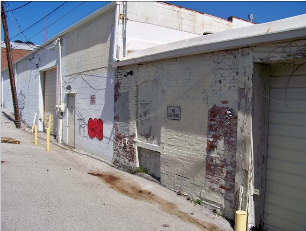
3634-3636 Main St – looking northeast – graffiti
