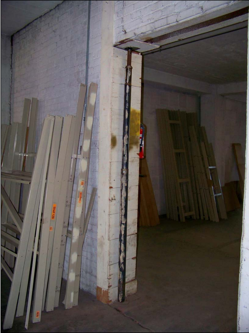
3244 Main St – interior – deterioration of lintels; cracking of wall, floor
