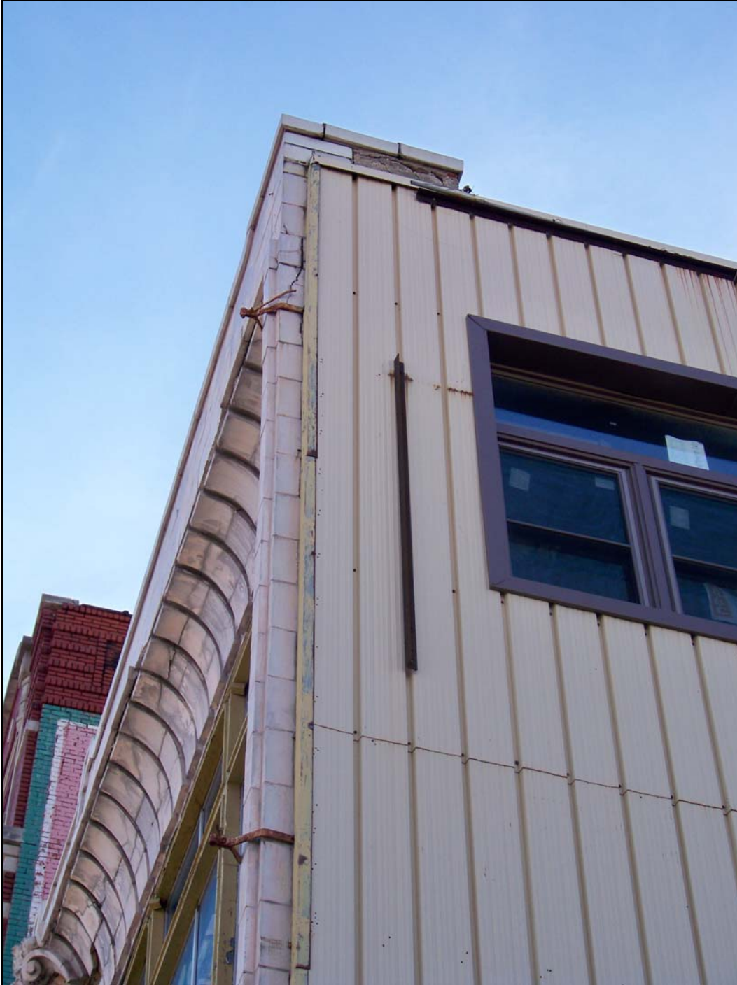
3240 Main St – looking southwest – deterioration of terra cotta; failure of finishes
