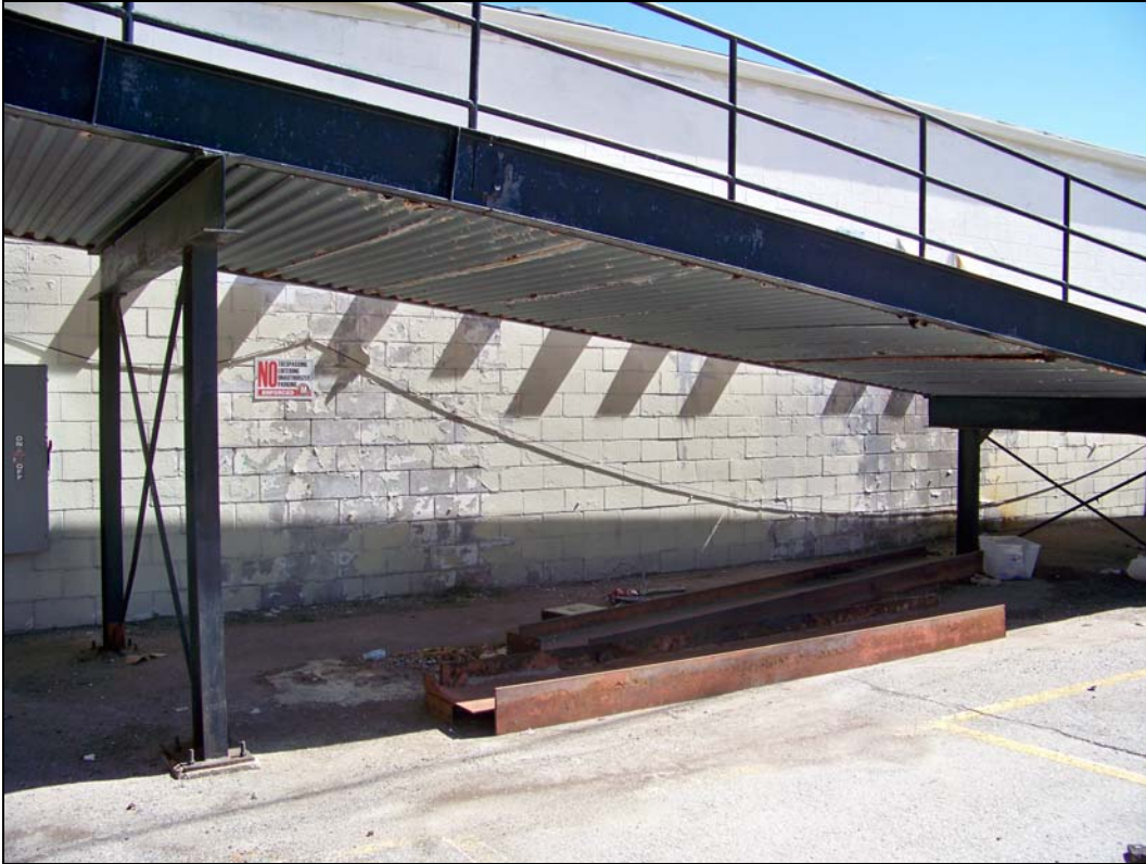
3634 Main St – looking east – failure of finishes; corrosion of ramp structure
