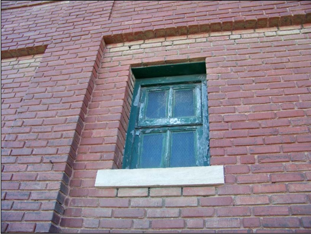
3244 Main St – looking west – failure of finishes
