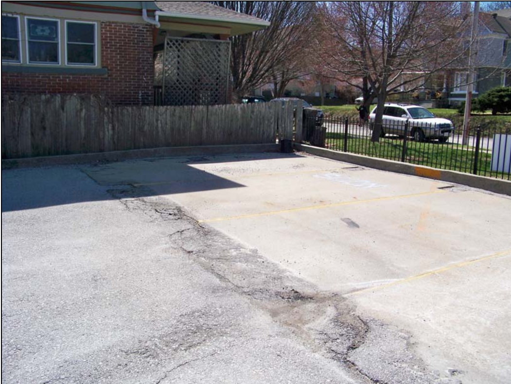
3635 Baltimore Ave – looking south – deterioration of pavement
