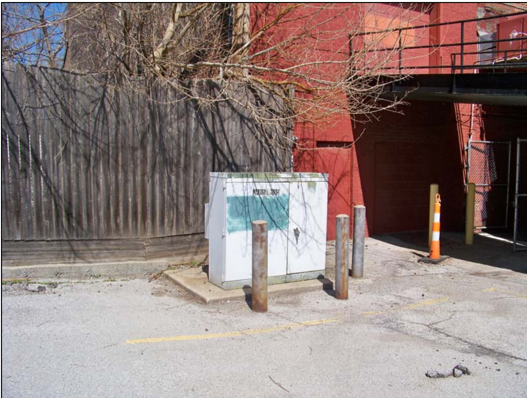
3633 Baltimore Ave – looking north – failure of finishes; deterioration of pavement
