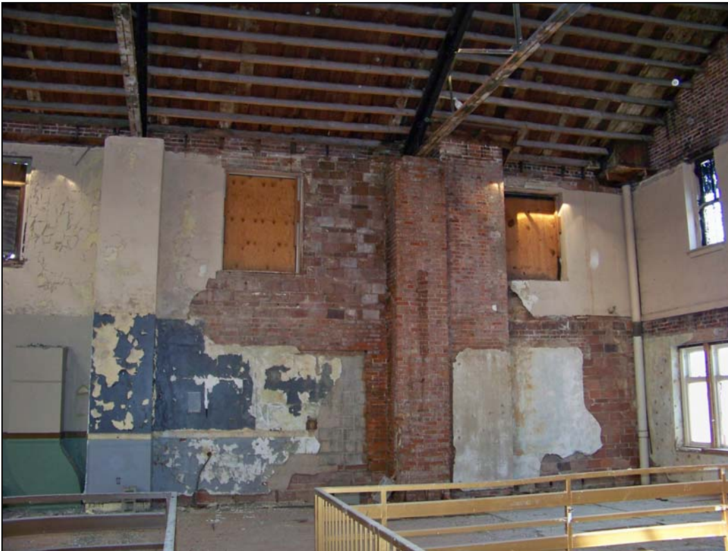
3620 Main St – interior – deterioration of windows; failure of finishes
