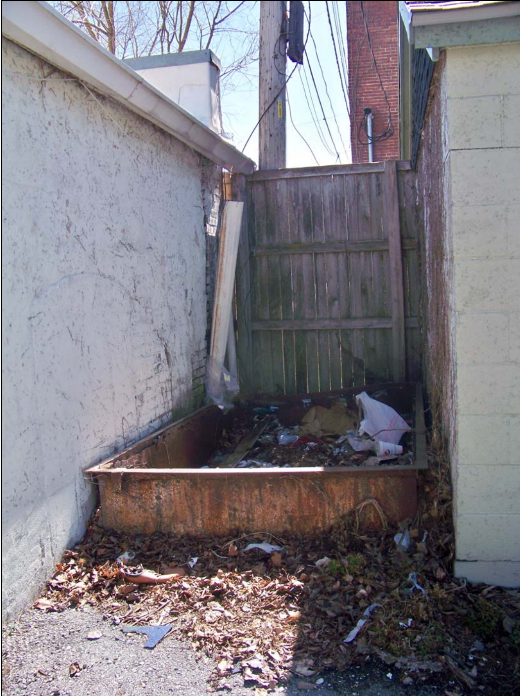
3636 Main St – looking south – deterioration of downspout
