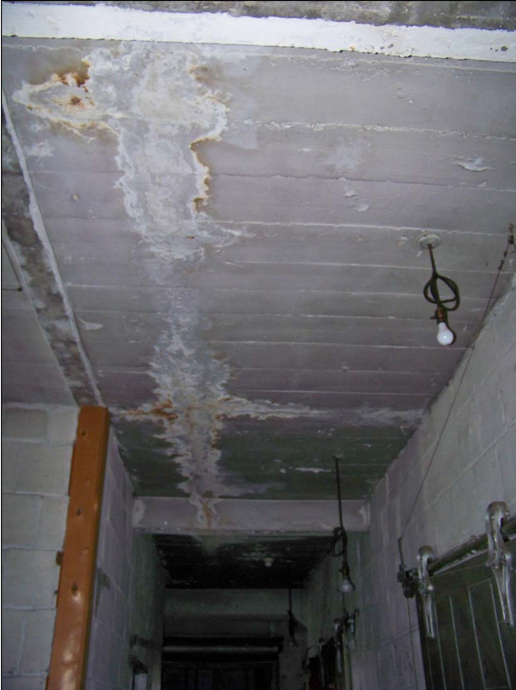
3244 Main St – interior – deterioration of concrete structure; water damage, corroding steel rebar
