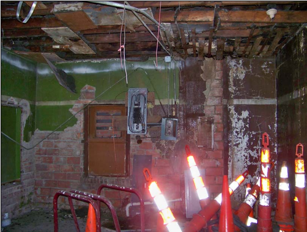
3634 Main St – interior – inoperable building system; deterioration of ceiling, wall coverings, finishes
