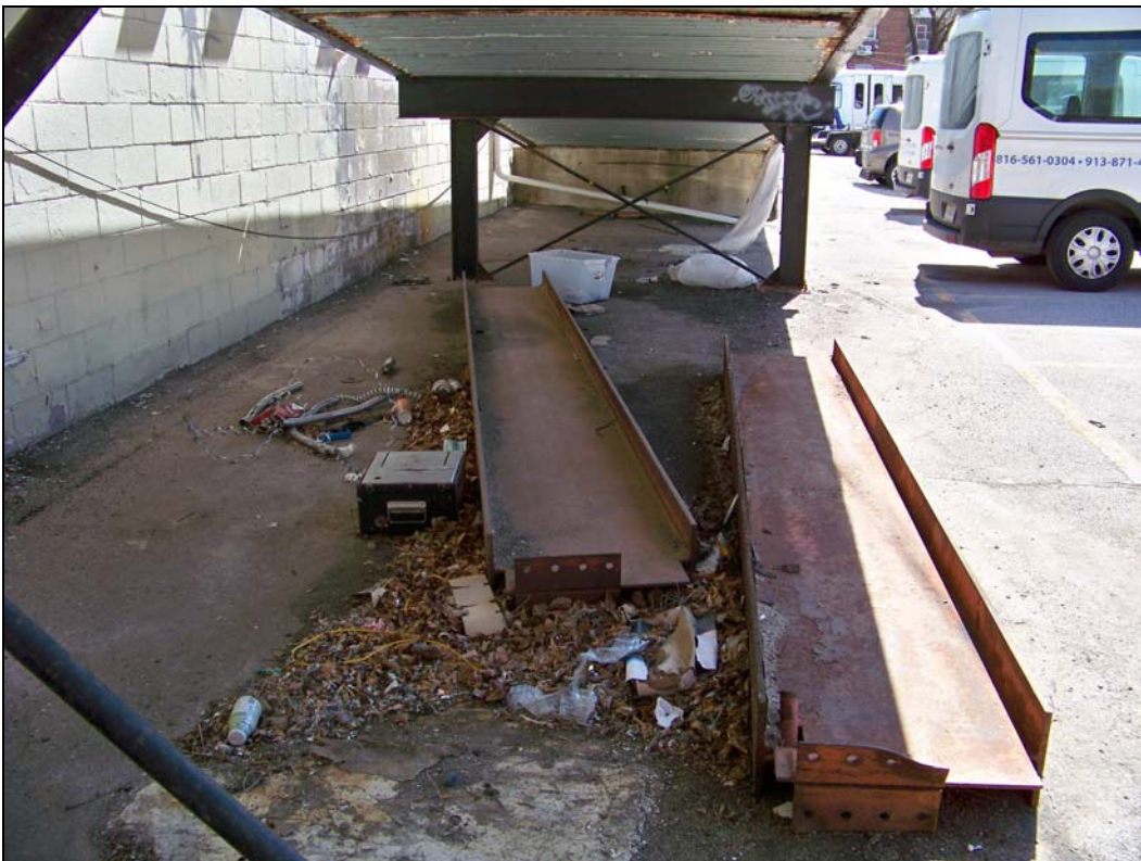
3634 Main St – looking south – trash/debris
