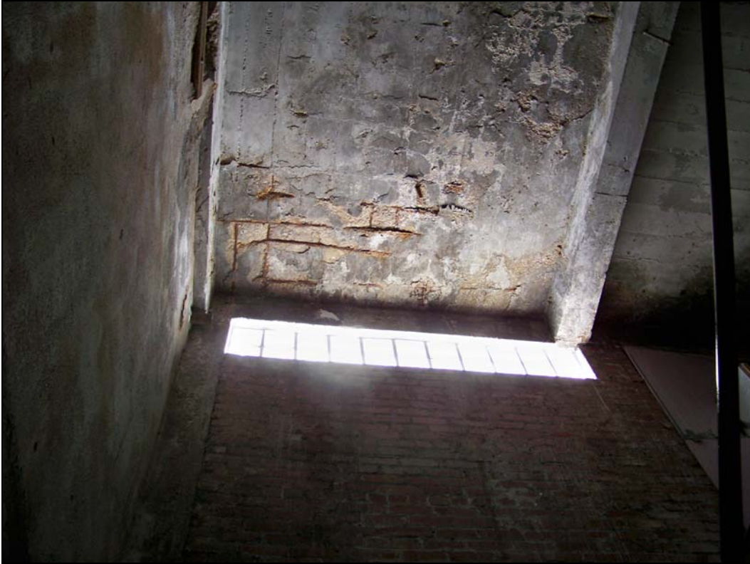
3240 Main St – interior – deterioration of concrete structure
