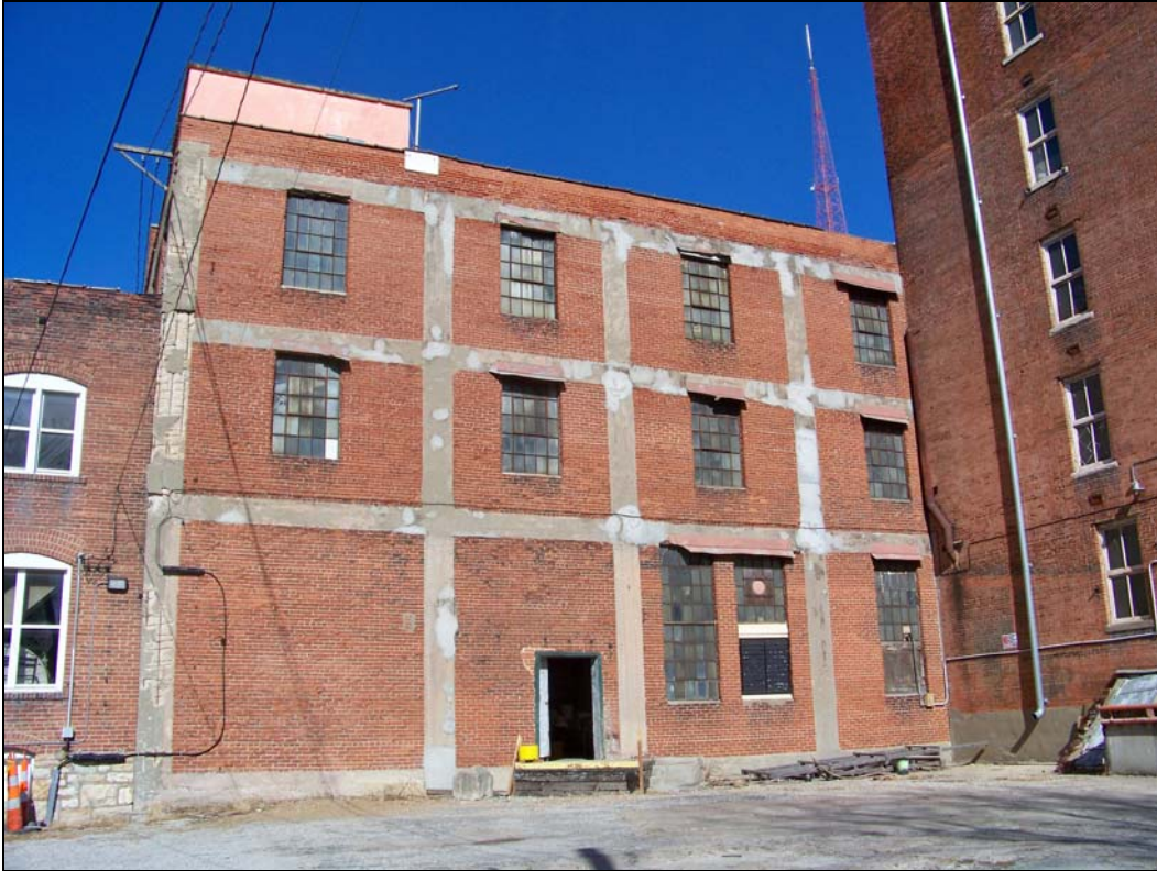
3240 Main St – looking north – deterioration of windows, concrete structure
