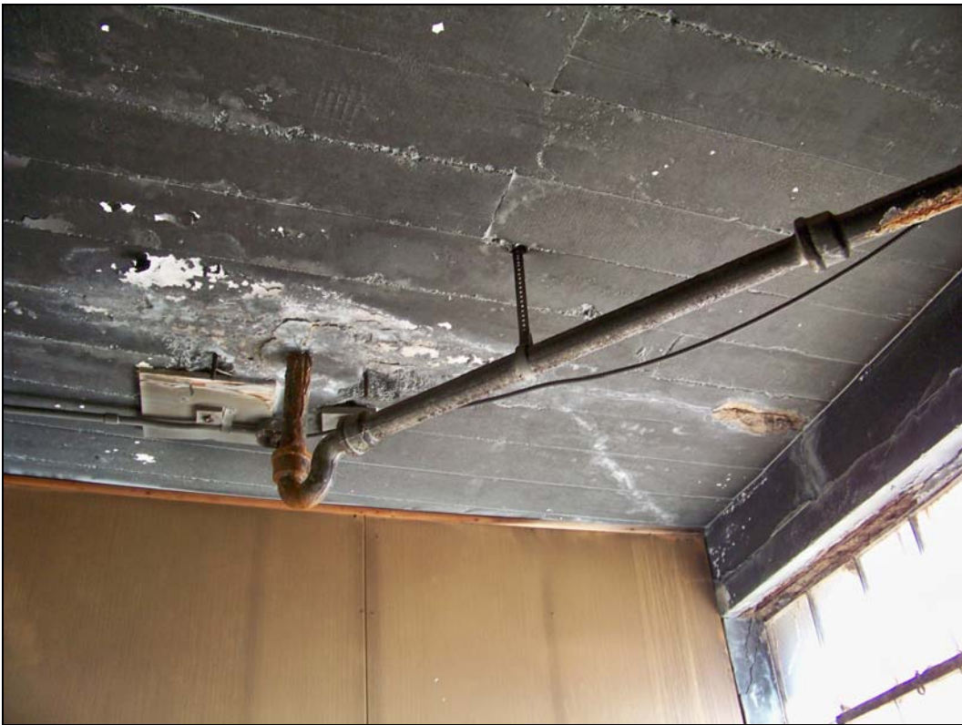
3240 Main St – interior – deterioration of window, concrete structure, plumbing
