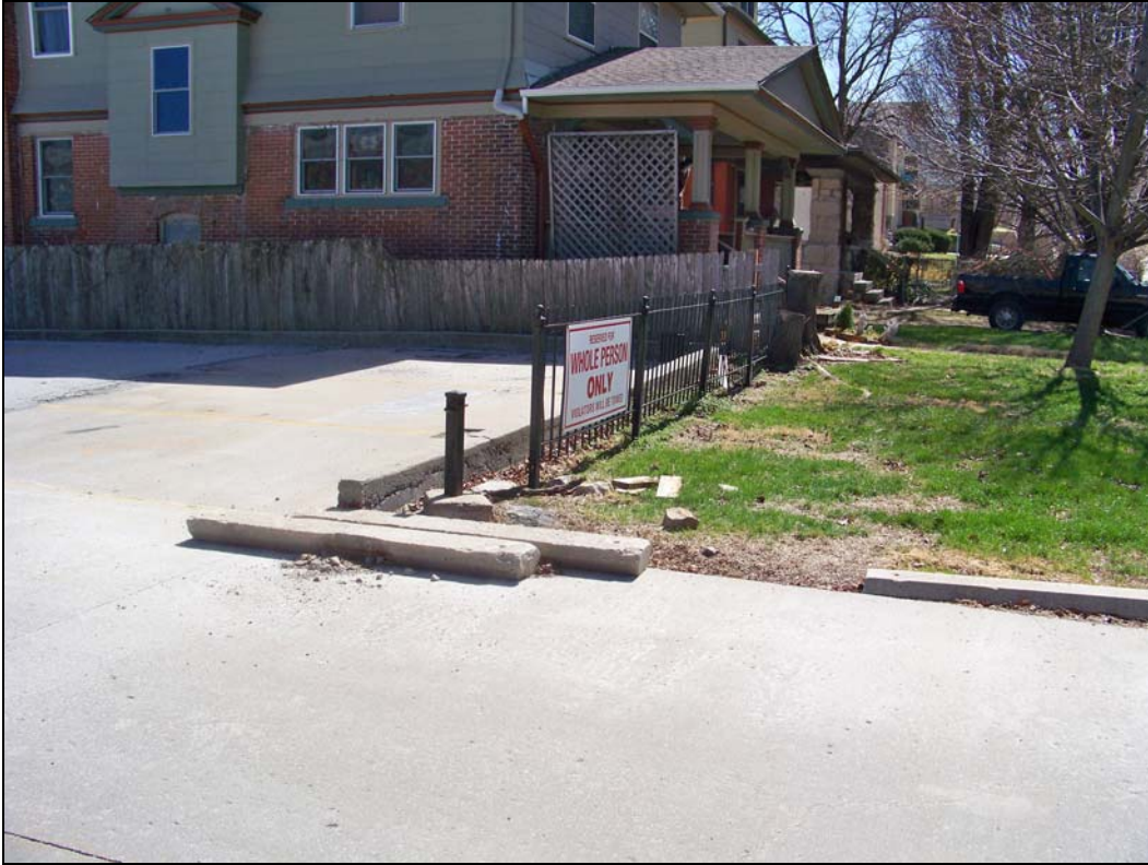
3635 Baltimore Ave – looking south – trash/debris
