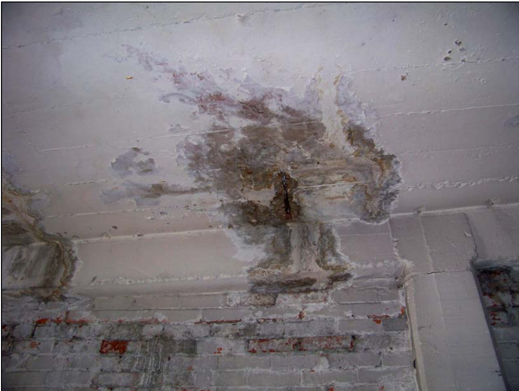
3244 Main St – interior – deterioration of concrete structure; water damage, corroding steel rebar
