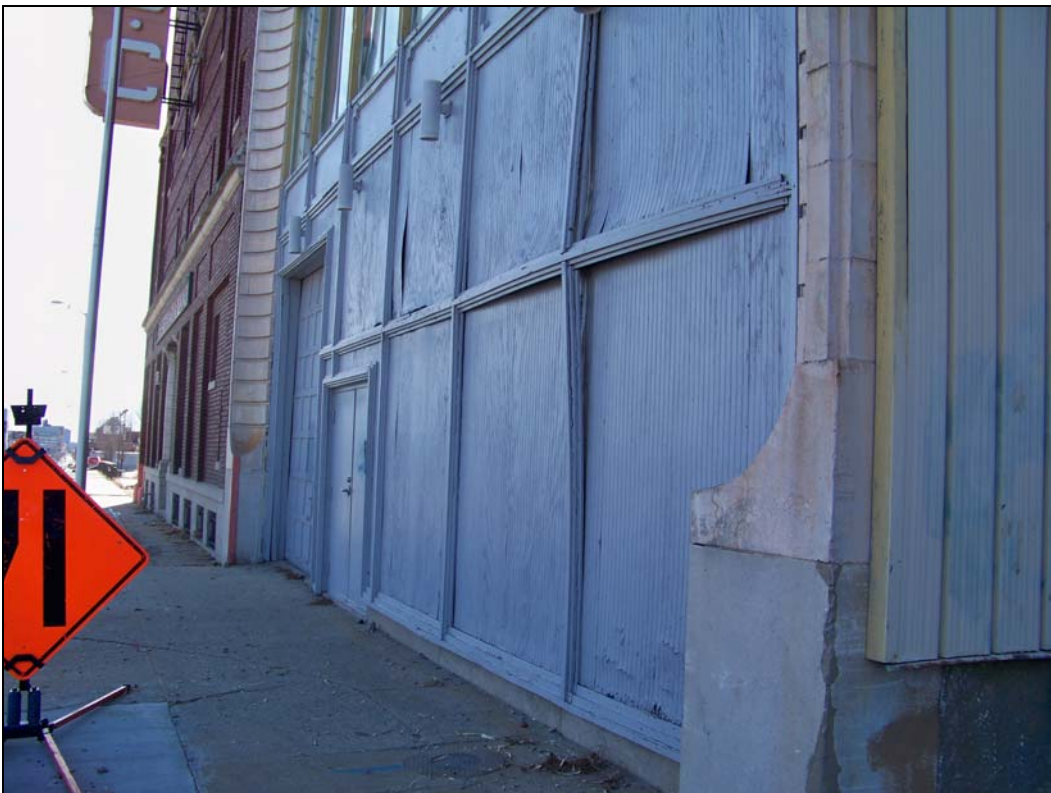
3240 Main St – looking south – deterioration of wall; failure of finishes
