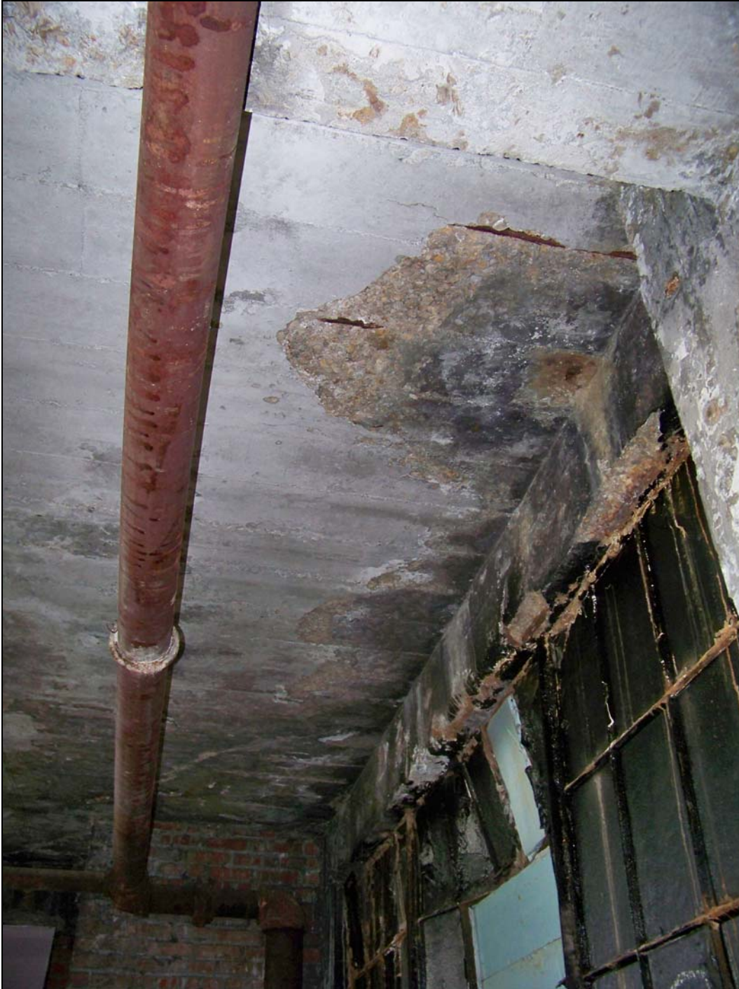
3240 Main St – interior – deterioration of window, concrete structure, plumbing
