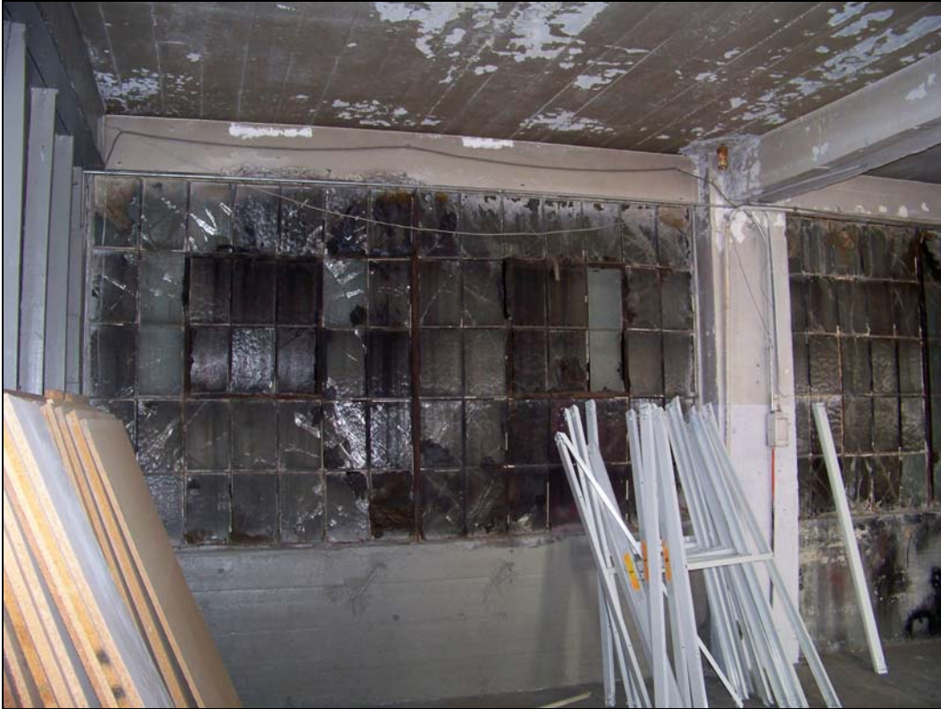
3240 Main St – interior – deterioration of windows, concrete structure
