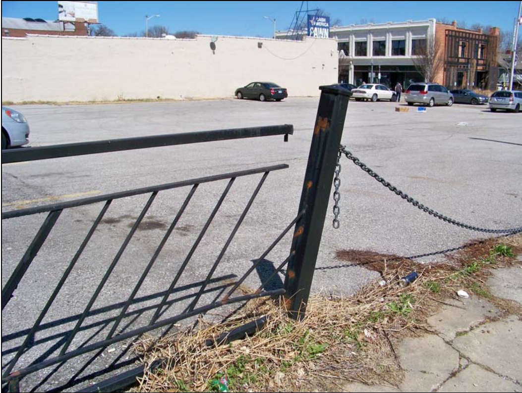
2 W. 37 th St – looking north – deterioration of fence, sidewalk
