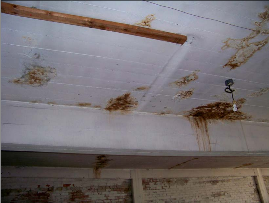
3244 Main St – interior – deterioration of concrete structure; water damage, corroding steel rebar
