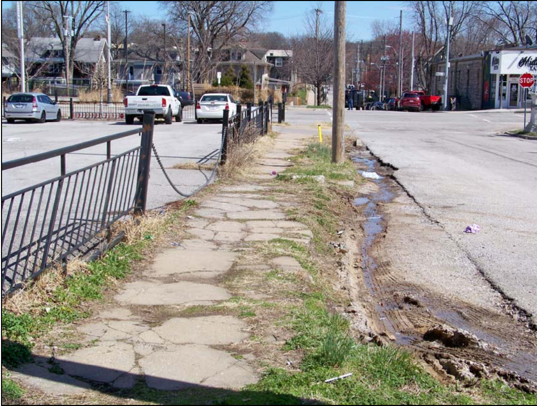
2 W 37 th St – looking east – cracked/uneven sidewalk and curb
