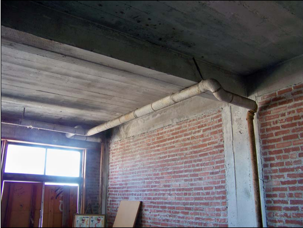
3244 Main St – interior – asbestos pipe-wrap
