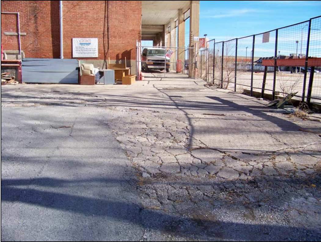
3244 Main St – looking east – deterioration of pavement
