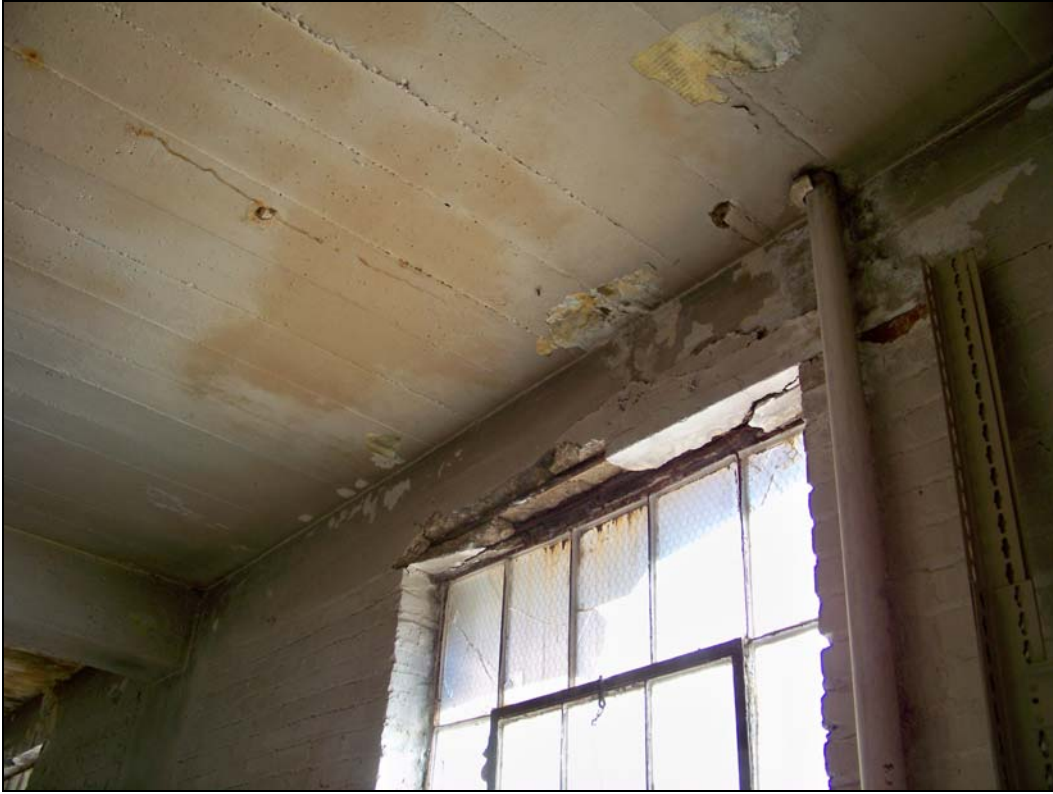
3240 Main St – interior – deterioration of window, concrete structure
