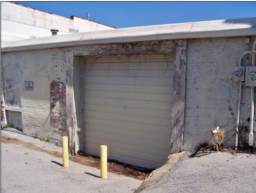
3636 Main St – looking east – failure of finishes
