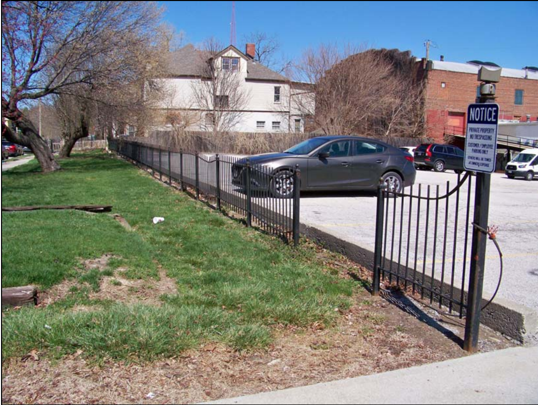
3635 Baltimore Ave – looking north – deterioration of fence
