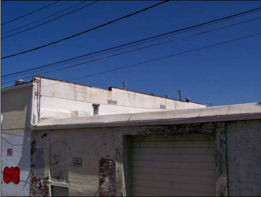
3634-3636 Main St – looking north – deterioration of roof coping; failure of finishes
