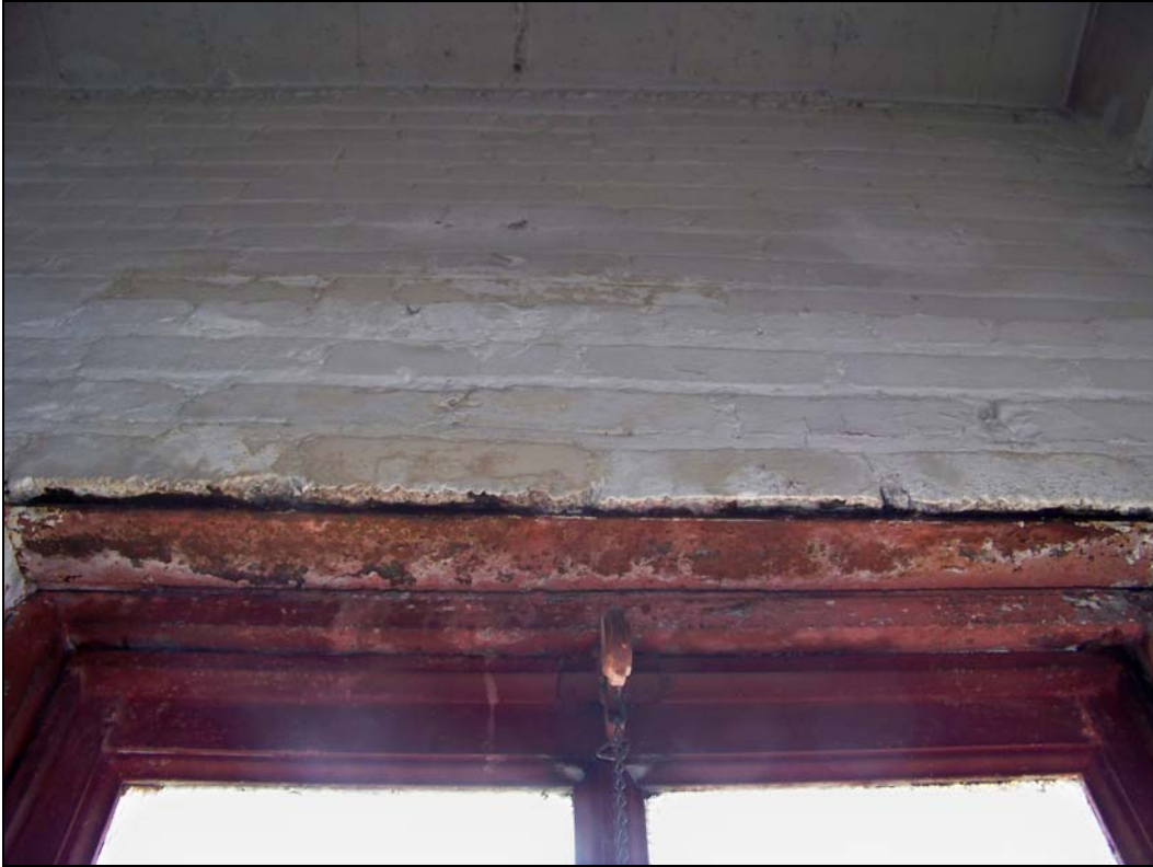
3244 Main St – interior – deterioration of window, lintel; failure of finishes
