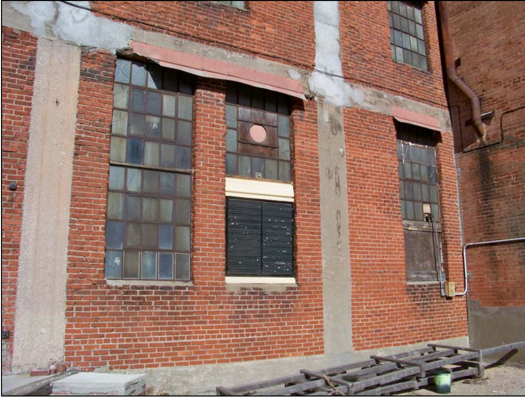
3240 Main St – looking north – deterioration of windows, concrete structure, venting
