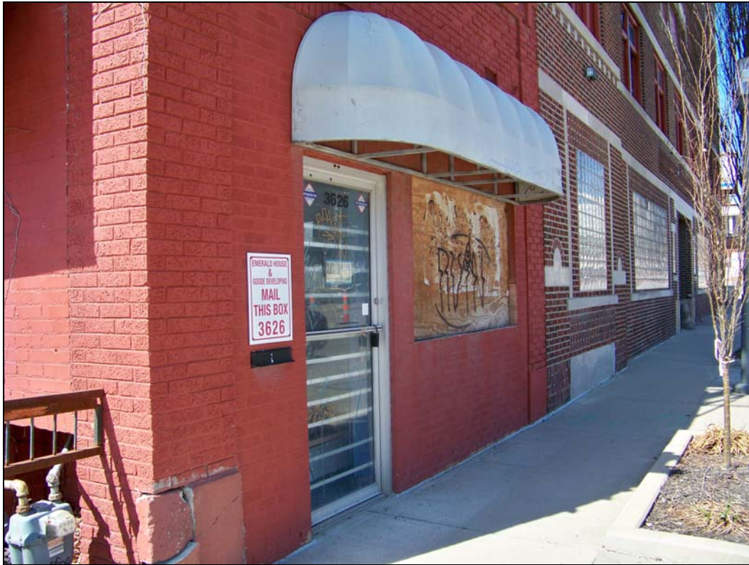
3626 Main St – looking northwest – deterioration of window
