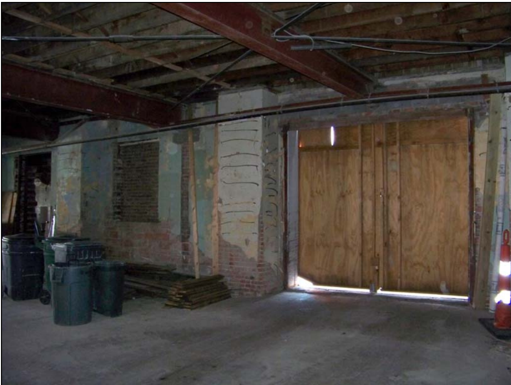
3620 Main St – interior – deterioration of door; failure of finishes
