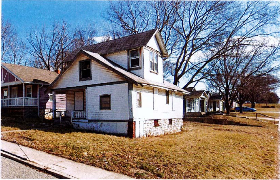
2031 E. 24 th Terrace – note broken and boarded windows, deteriorated soffits and eaves
