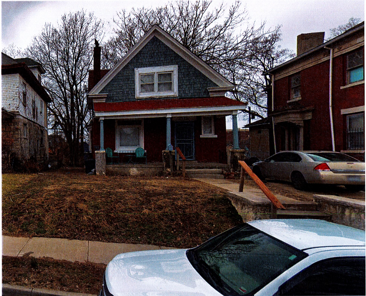
2538 Park Avenue – note porch roof tilting to left, failing surface treatments
