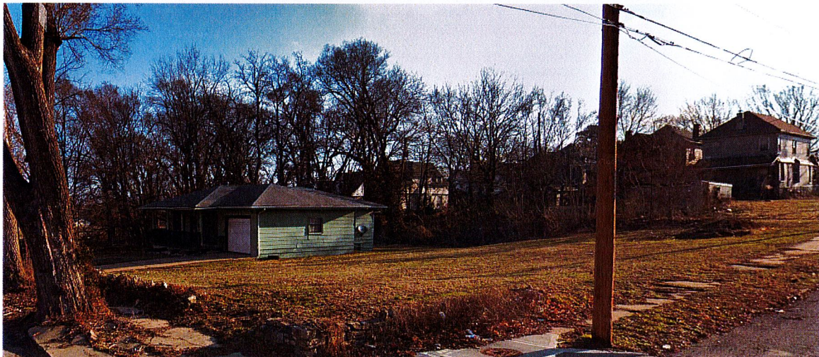
2400 – 2404 E. 25 th Street – note broken sidewalks, deteriorating retaining wall, overgrown brush
