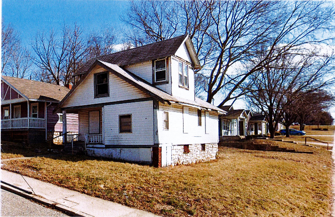
2031 E. 24 th Terrace – note broken and boarded windows, deteriorated soffits and eaves
