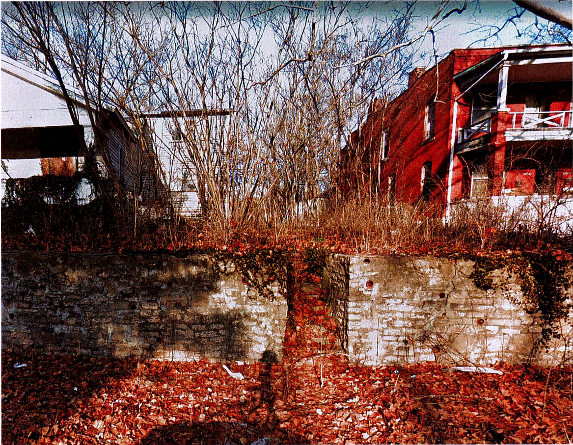
2317 Olive – note deteriorating retaining wall and stairs, overgrown brush and trees
