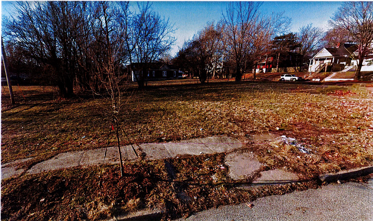
2404 – 2406 E. 23 rd Street – note broken and missing sidewalk and driveway apron, recently cleared
