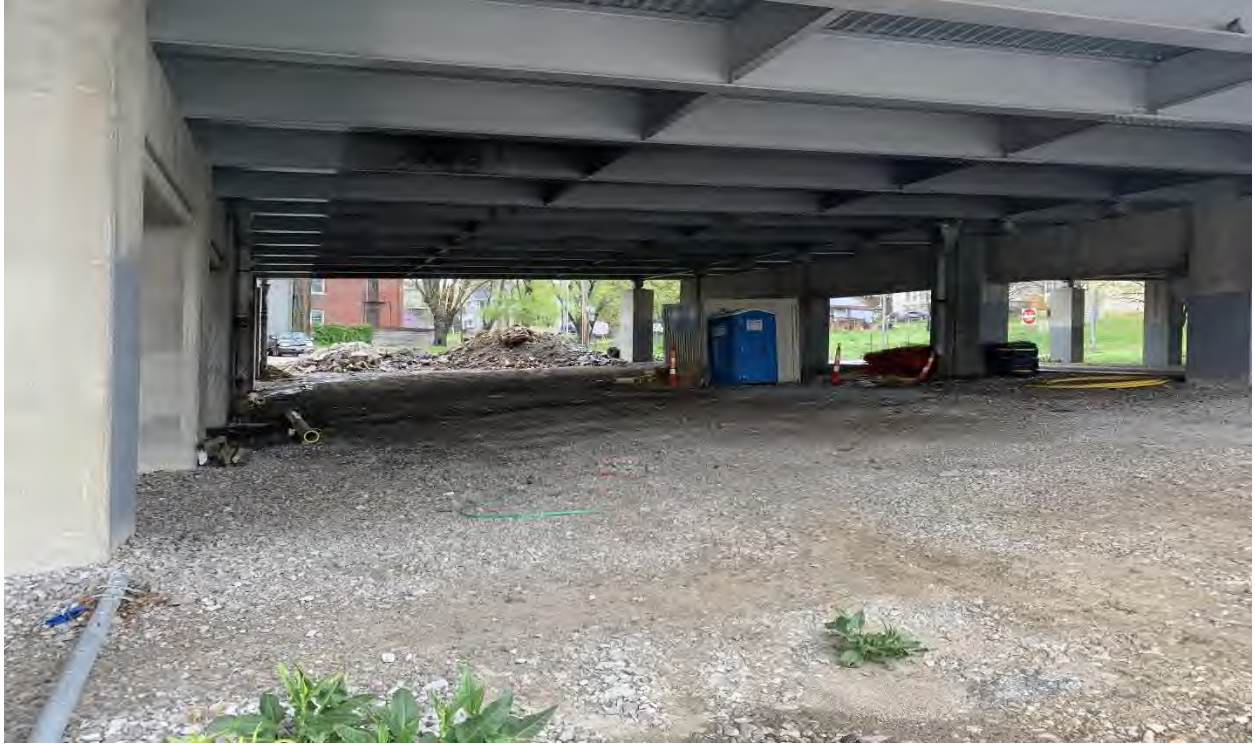
Figure 17. Underpass at Pennsylvania south of 20th St. Graffiti and debris.
