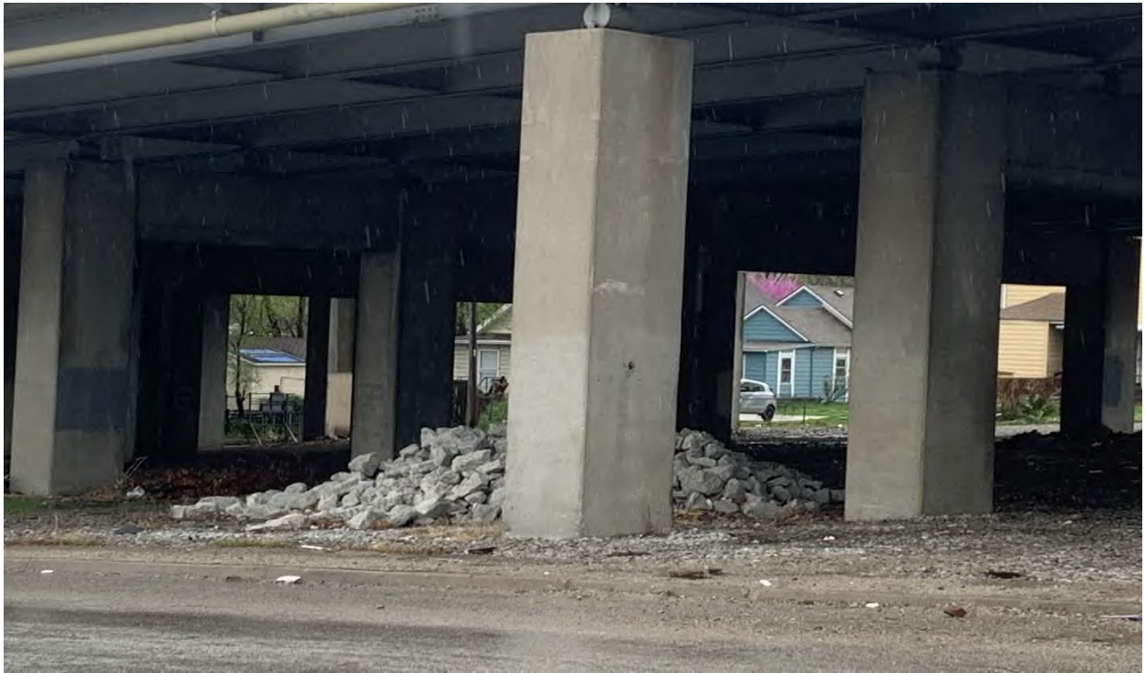
Figure 19. Pennsylvania south of 20th. Loose and broken concrete.
