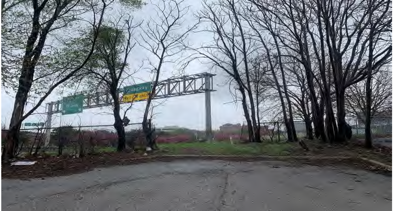
Figure 1. Far end of Washington Street from 17th Street. Safety fence missing, leading to the freeway.
