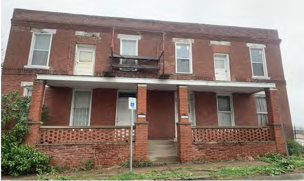
Figure 5. 802 W. 16th St. House in disrepair.
