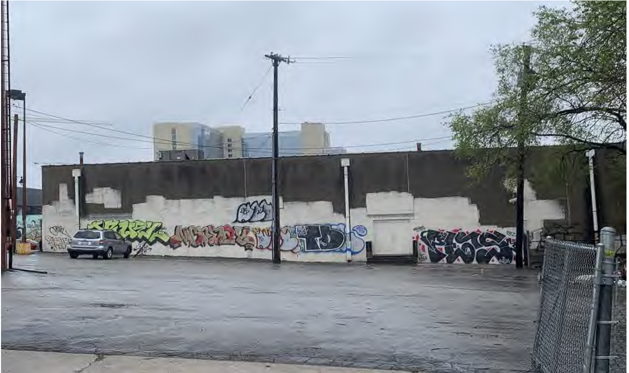
Figure 16. 1616 Broadway Blvd. Graffiti to rear of building.
