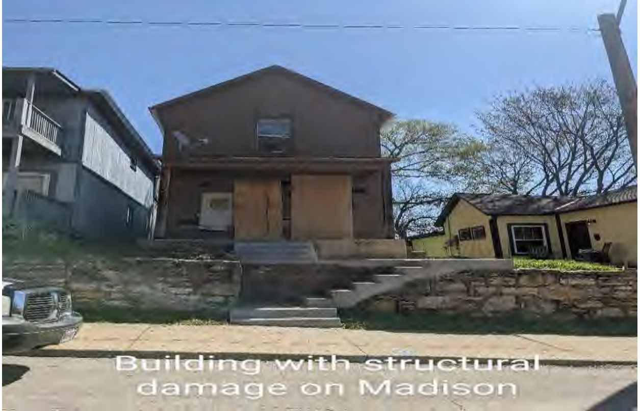
Figure 12. 2141 Madison Ave. Disrepair.
